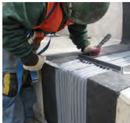
▼ MetLife Stadium Expansion Joints - Rutherford, NJ
